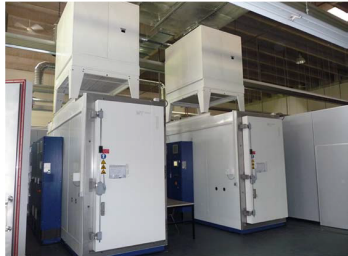
Machinery for Double Height Room in ISAAC
