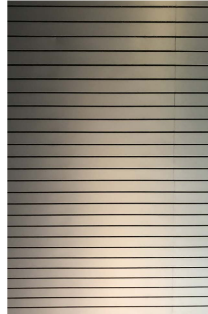
Aluminium hanged ceiling
