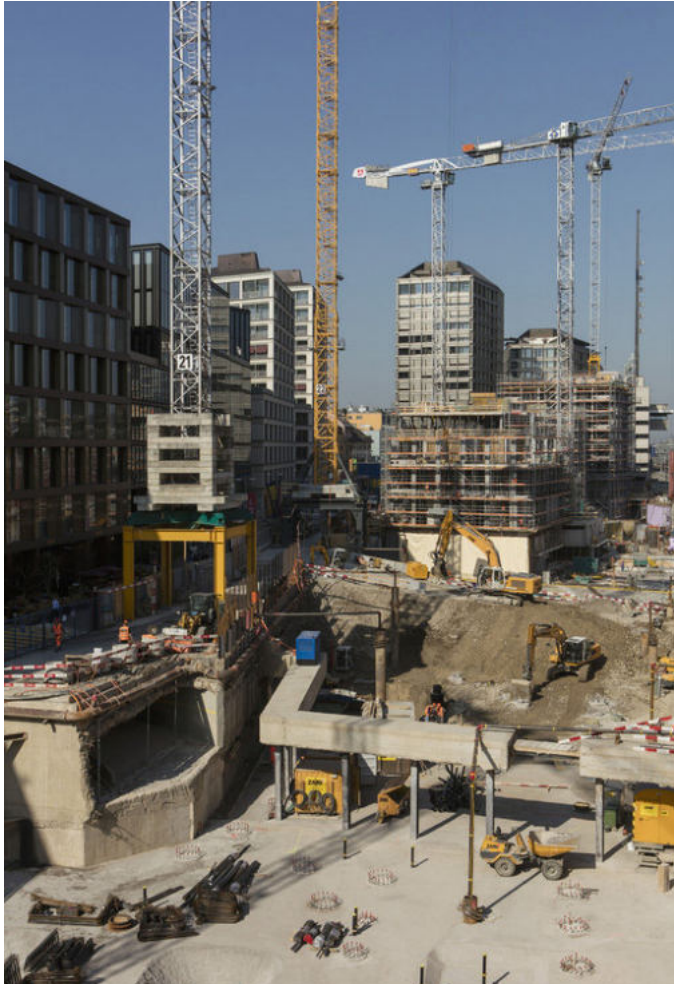
Figure 16 Moments inside of the foundation of plot D. Source: Wiel Arets Architects.
